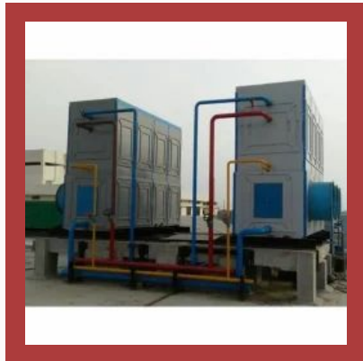
Ammonia Evaporative Condenser
