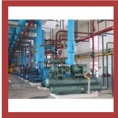
Ammonia Refrigeration Plants
