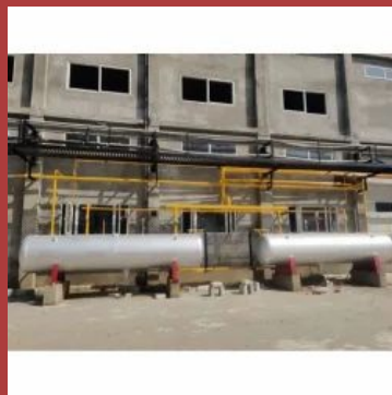
Ammonia Gas Storage Tank
