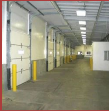
Potato Cold Storage Plant
